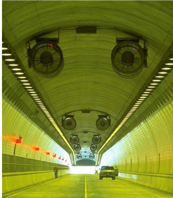
Figure 2-6 Ventilation System with Jet Fans at Cumberland Gap Tunnel
