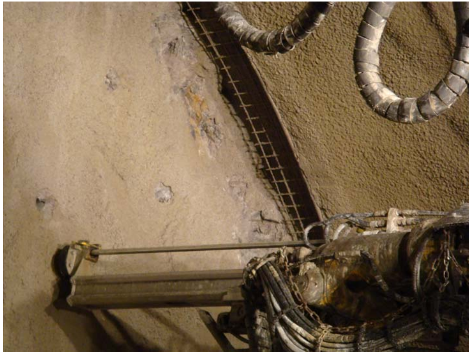
Figure 9-11 Shotcrete Lining Installed at the Face in a SEM Tunnel Excavated by Drill-and-Blast (Andrea Tunnel, Austria)
