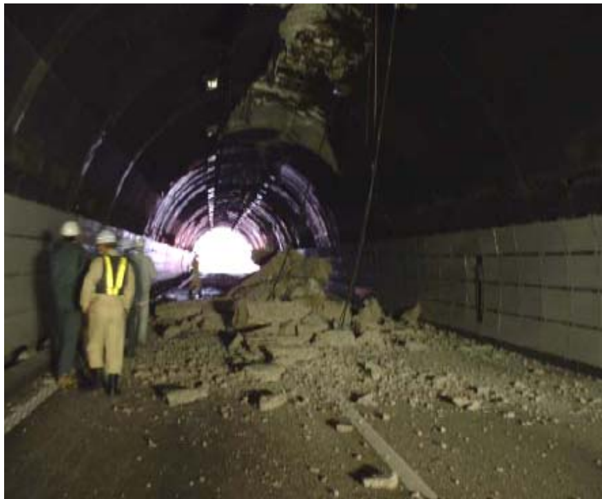
Figure 13-8 Highway Tunnel Lining Falling from Tunnel Crown – 2004 Niigata Earthquake, Japan
