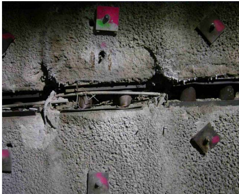
Figure 8-4 Yielding Support Crushed to 20 cm (One-half) (ILF, 2008)
