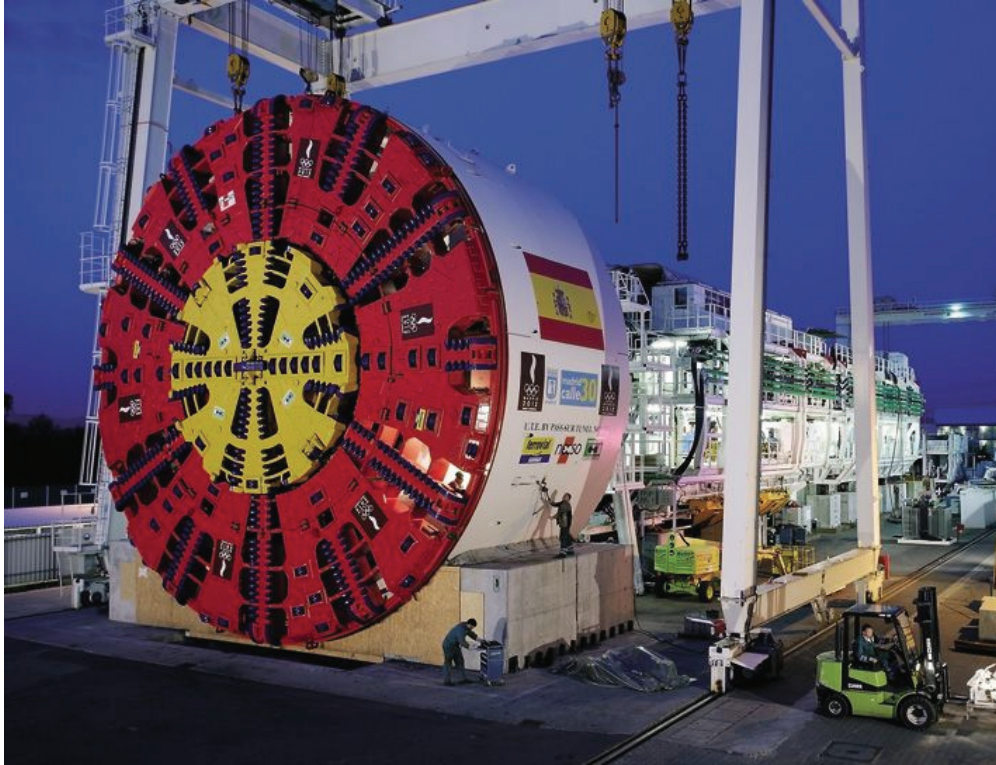
Figure D-11 The EPB Machine for the M30-By-Pass Sur Tunnel Norte project in Madrid.
