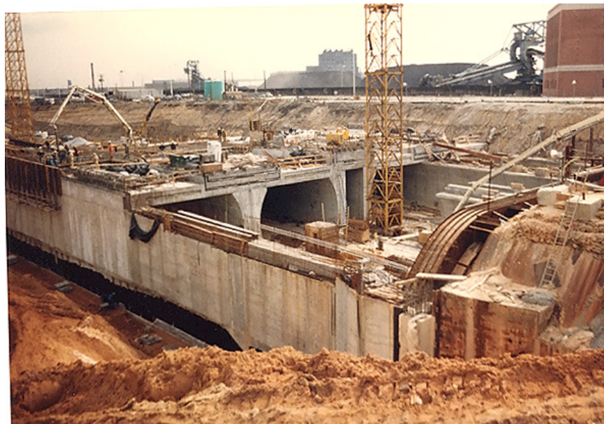
Figure 5-3 Cut and Cover Construction using Side Slopes Excavation- Ft McHenry Tunnel, Baltimore, MD
