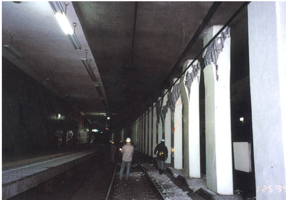
Figure 13-11 Shear Failure at Top of Columns of Cut-and-Cover Tunnel Between Daikai and Nagata Stations - 1995 Kobe Earthquake, Japan
