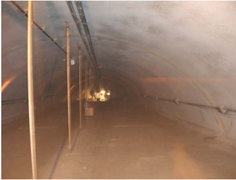
Figure 16-6 Negative Side Cementitious Coating, Tuscarora Tunnel PA Turnpike
